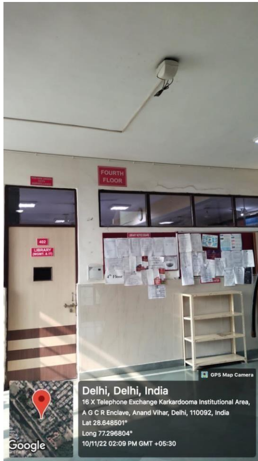
Fourth Floor, Wi-Fi Facility
