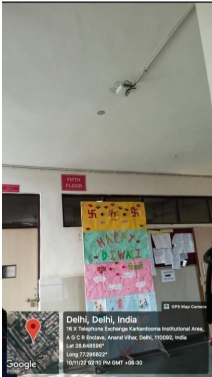
Fifth Floor, Wi-Fi Facility
