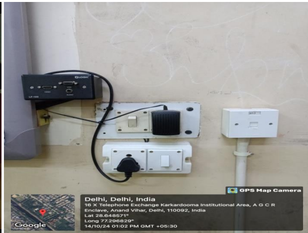
LAN Port in Classrooms
