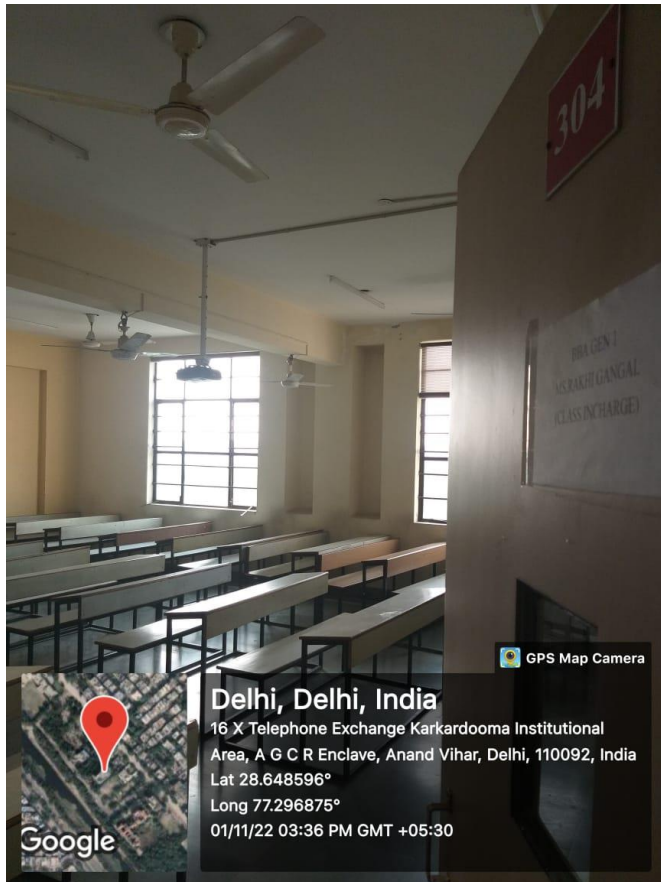
ROOM NO.304,WALL MOUNTED PROJECTOR
