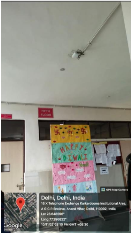
Fifth Floor, Wi-Fi Facility
